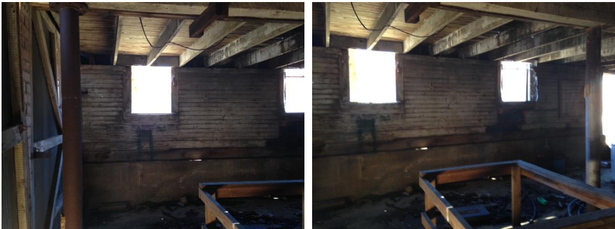
Two views of downstairs west wall with 12" thick concrete lower wall and wooden pony wall above. Note that the double hung sash windows are placed so that only the lower panes are visible from inside.
