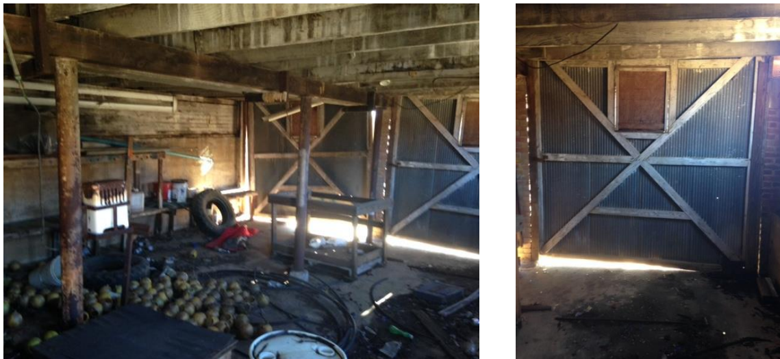
Downstairs has 70" high concrete foundation walls on the east, three iron center posts, & pulley-mount doors.
