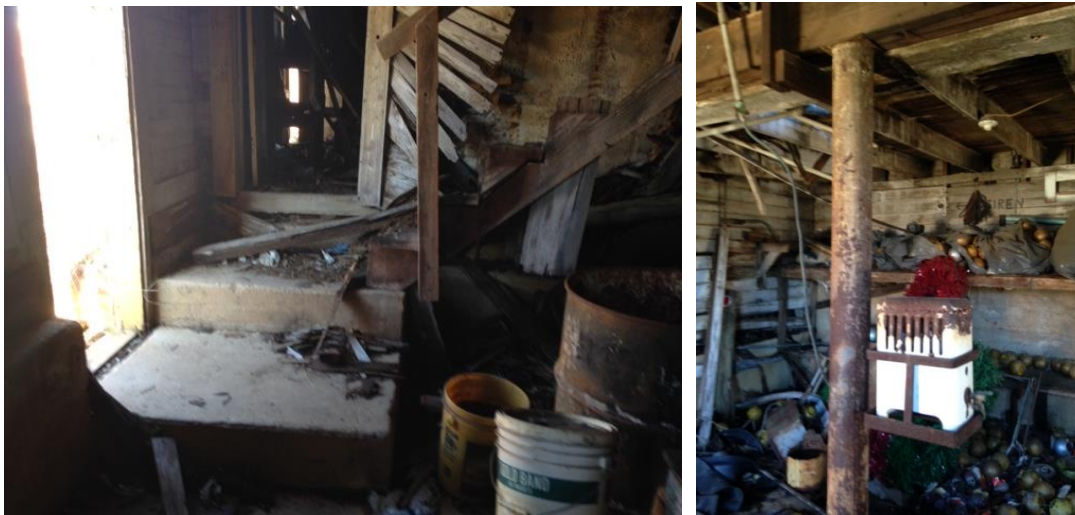
West side entrance landing (left) and middle iron post of lower level (right).
